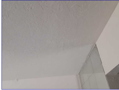
There is staining on the bedroom ceiling. No current moisture at the time of the inspection. Monitor and repair as needed.
