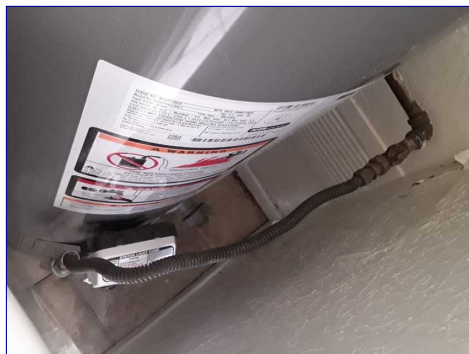
Gas line needs debris trap.
