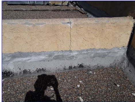
Parapet walls need repair,
