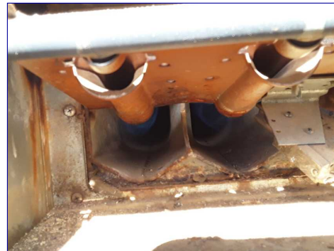
Orange flame on burners, should be blue.
