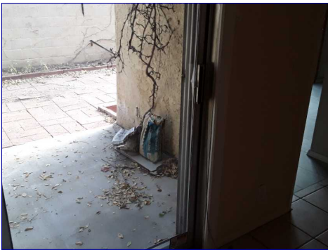
Latch was broken door wasn't latching.
