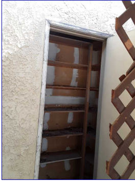
The exterior trim was in need of normal painting maintenance. Recommend a professional painter repair/paint the exterior trim.
