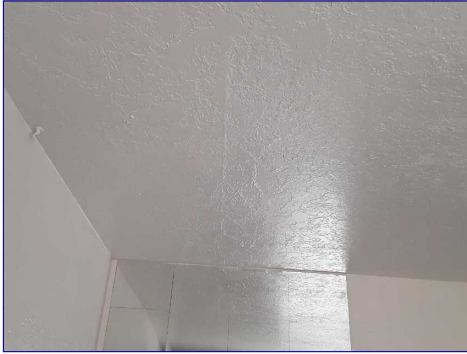
There is staining on the bedroom ceiling. No current moisture at the time of the inspection. Monitor and repair as needed.
