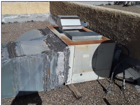
Furnace was not evaluated. Recommend an HVAC contractor evaluate.
