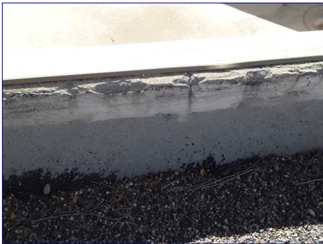
Parapet walls need repair,
