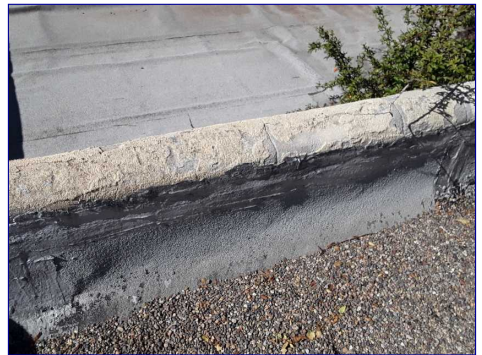
Parapet walls need repair,
