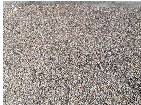
Soft spot on roof.
