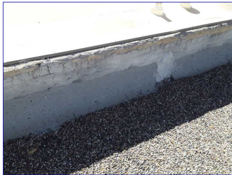
Parapet walls need repair,
