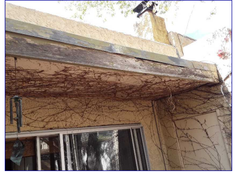
The exterior trim was in need of normal painting maintenance. Recommend a professional painter repair/paint the exterior trim.
