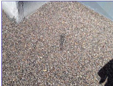
The roof is considered marginal and requires repair. Recommend a licensed contractor repair all affected areas.
