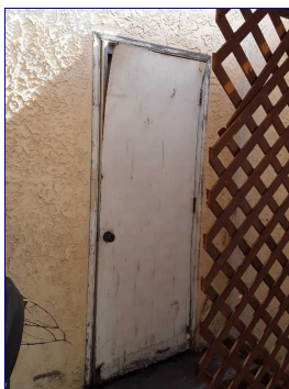
Storage room door need replacement.
