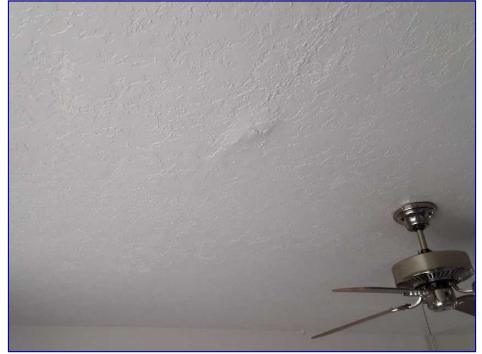
There is staining on the bedroom ceiling. No current moisture at the time of the inspection. Monitor and repair as needed.
