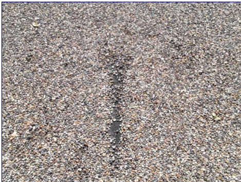
The roof is considered marginal and requires repair. Recommend a licensed contractor repair all affected areas.
